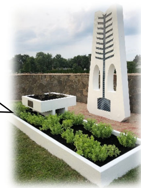
← Before and After → Repairs made by Masotti Construction to the Hurwitz Memorial Wall
